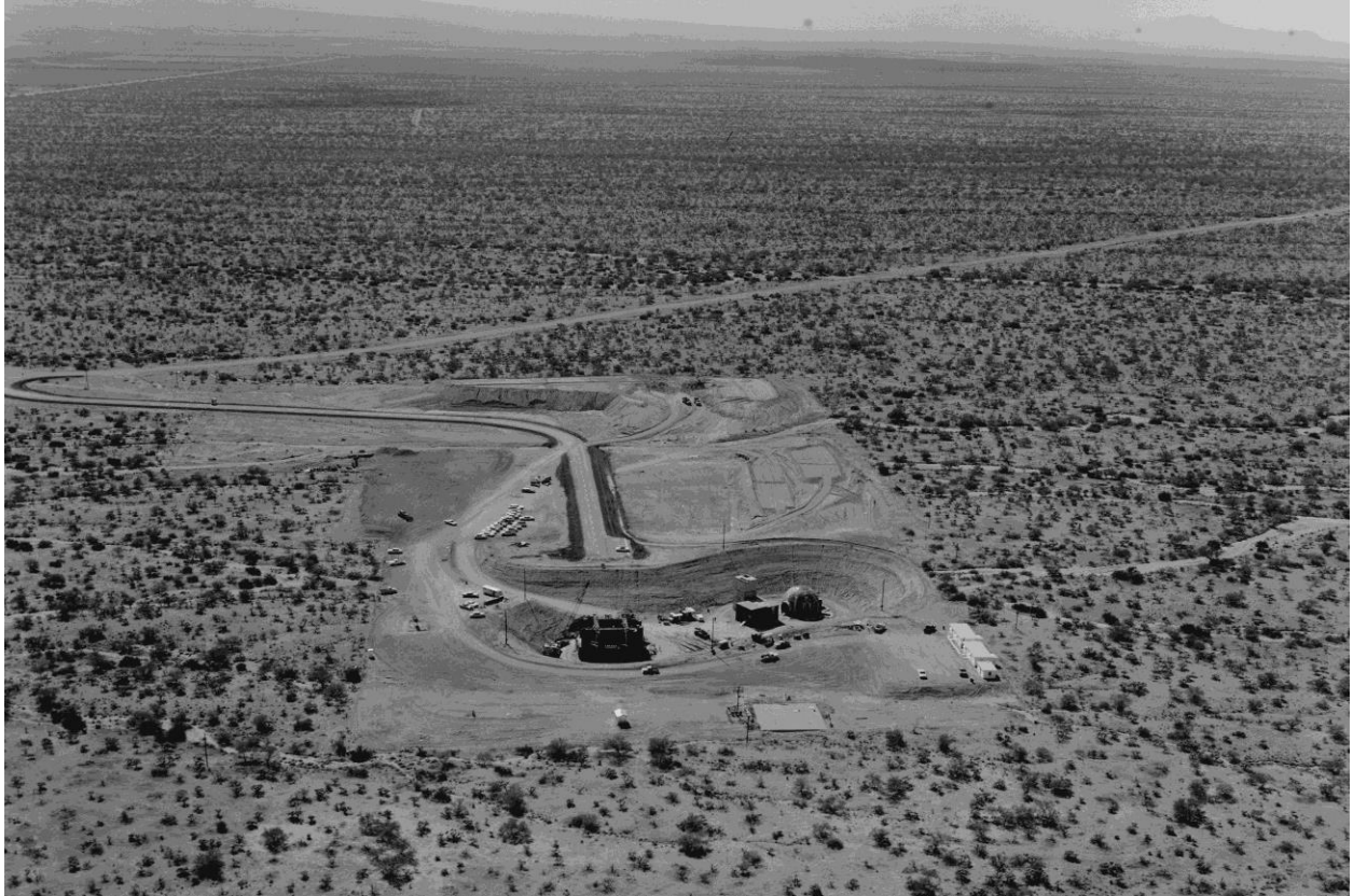
Missile site 571-7 under construction in 1962. The silo cover is seen at the left side of excavation, with the blast lock and control center to the right.
