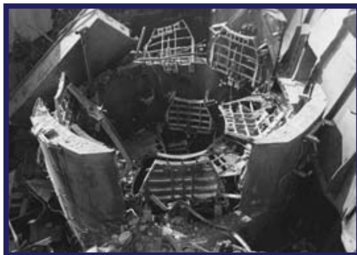
A close-up view at the silo ruins. Damaged beyond repair.
