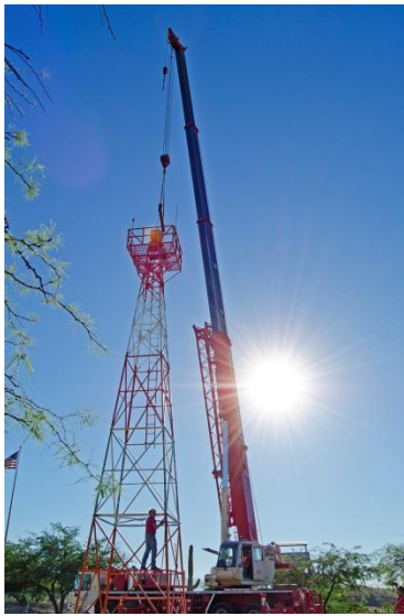
PASMBeaconCrane.jpg = crane moving the beacon to its new location near Valencia Rd. during the early morning. Photo by Andrew Boehly
